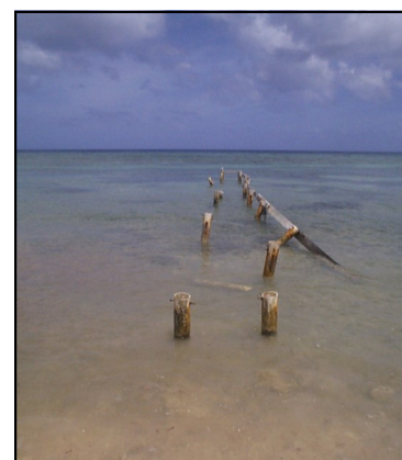
Photo 4: Removal may be necessary if a damaged dock is creating a navigational hazard. The Port Authority can advise on this. A Coastal Works Permit is required for works on the seabed.
